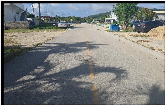
NEW ASPHALT ROADWAY AND LOCATION OF THE NEW INSTALLED SEWER MANHOLE 1 GOING TO SAN JOSE CHURCH ALONG APENGAGH STREET. (GOING NORTH).
