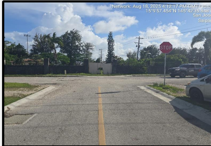
NEW ASPHALT ROADWAY AND THE START OF THE PROJECT LOCATED AT THE BACK OF BEST DEAL MERCHANDISE ALONG APENGAGH STREET (GOING SOUTH).
