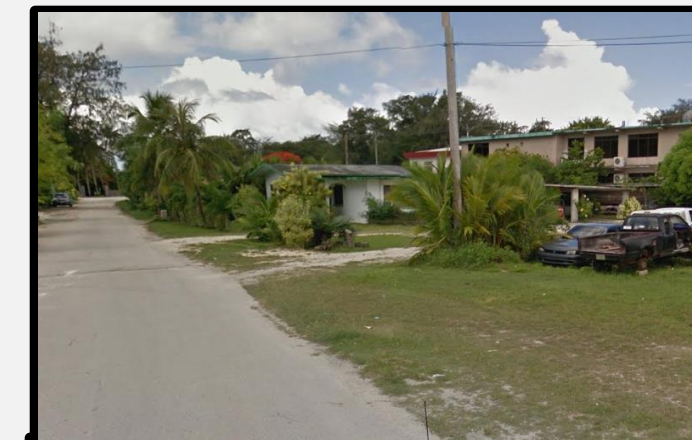
END OF THE PROJECT CONNECTING THE OLD AND NEW INSTALLED SEWER MANHOLE ALONG APENGAGH STREET (GOING SOUTH).
