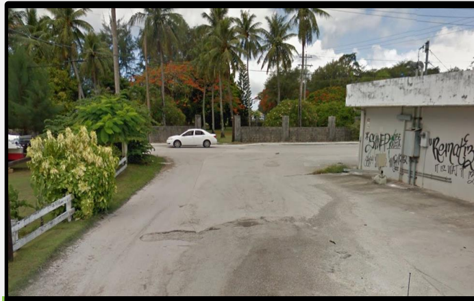
OLD ASPHALT ROADWAY AND THE STARTING POINT OF THE PROJECT AT THE BACK OF BEST DEAL MERCHANDISE ALONG APENGAGH STREET (GOING SOUTH)
