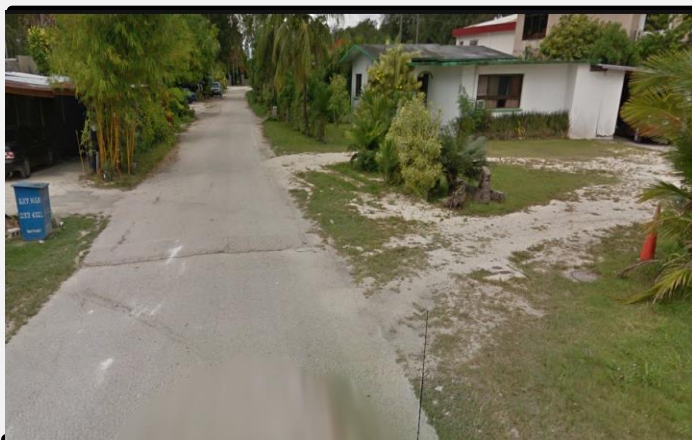
OLD ASPHALT ROADWAY AND LOCATION OF THE EXISTING SEWER MANHOLE 1 AT THE BACK OF NEW DOWNTOWN MARKET ALONG APENGAGH STREET (GOING SOUTH).
