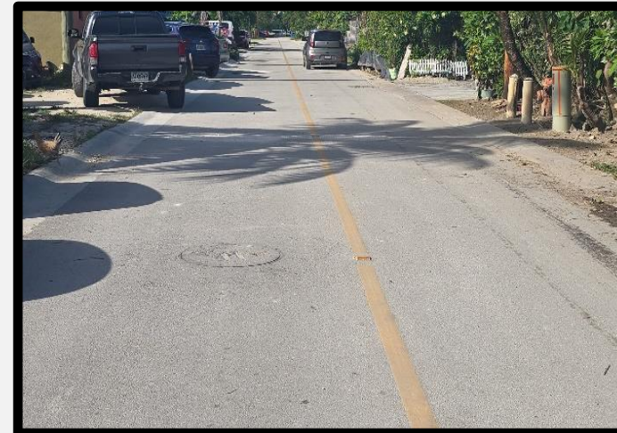
LOCATION OF THE NEW INSTALLED SEWER MANHOLE CONNECTED TO THE EXISTING SEWER MANHOLE 2 GOING TO SAN JOSE CHURCH ALONG APENGAGH STREET. (GOING NORTH).
