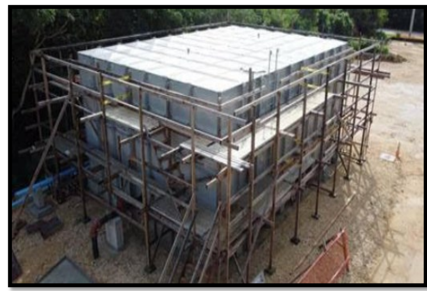
Dandan Temporary Water Tank
